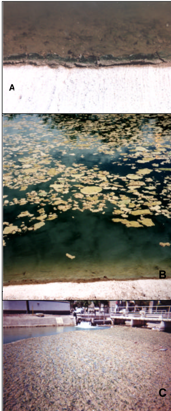
Figure 3.9. Periphyton mats grown along the submerged Arizona canal walls (A); detached floating algal mats (B); and accumulation of algal mats at a radial gate (C).
