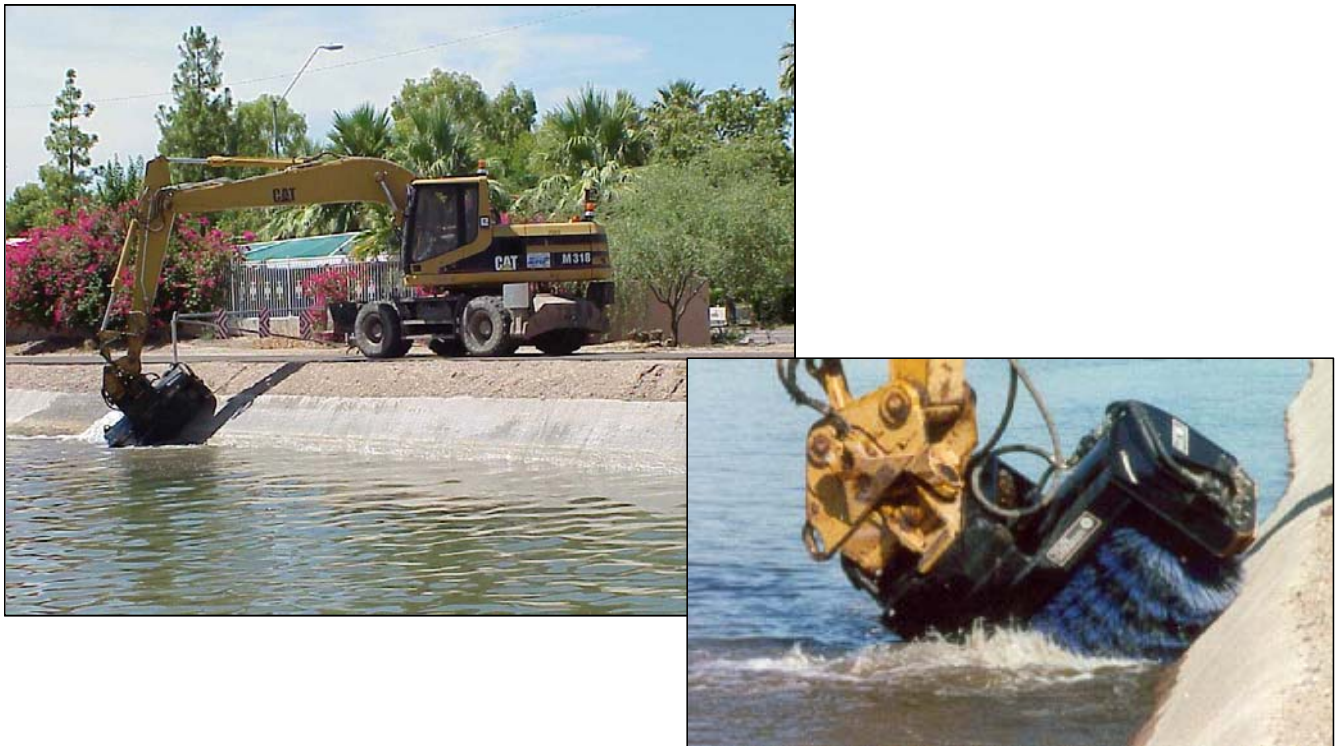
Figure 2.16 CAP and SRP canal devices for algae removal
